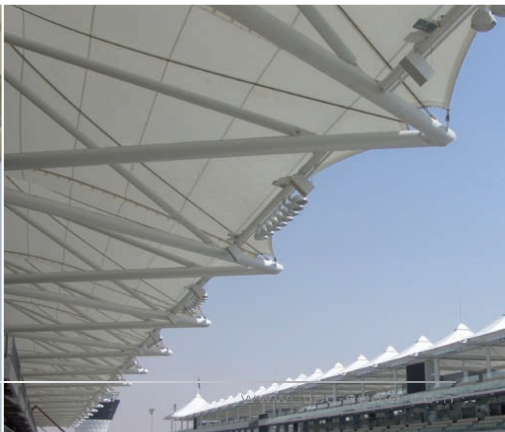
Roof of a grandstand with multiple speaker systems mounted at the front side edge
